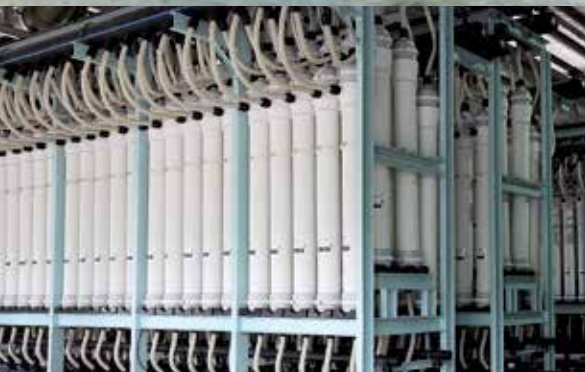
Above: Tuaspring Desalination Plant
