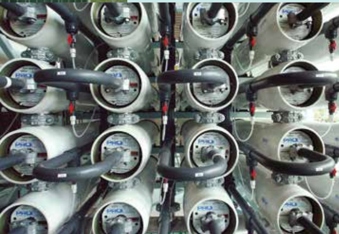
Below: Reverse osmosis membranes at the NEWater factory
