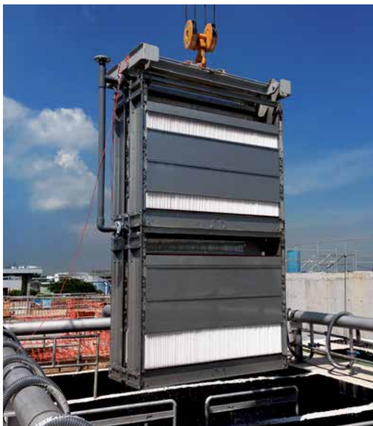
UASB-MBR demonstration plant at the Jurong Water Reclamation Plant.
