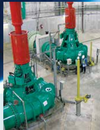
Above: The Influent Pumping Station located 60 m below ground at the Changi Water Reclamation Plant, implemented under DTSS Phase 1.
